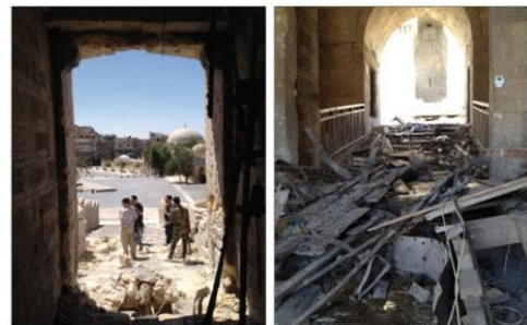
Fig. 8- Damage of Aleppo Citadel gate (SANA 2012)
