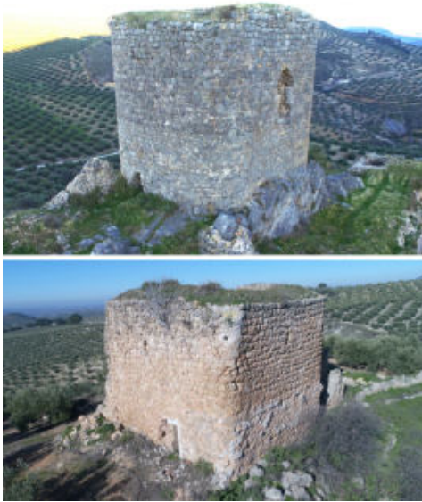
Fig. 5- Aerial views of the rounded corners of the keep tower of the fortresses of Víboras and Cortijo de la Torre (photos by the authors)
