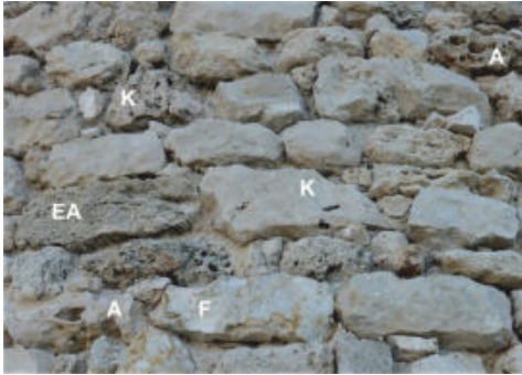
Fig. 5- Decay forms on the tower masonry. A= alveolation; EA= elongated alveolation (fissure); F= fracturing and flaking; K= karstification, (graphic elaboration by Fancello, 2022)
