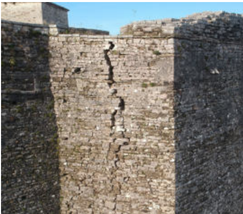
Fig. 4- Tower A cracks (Eppich, 2020)
