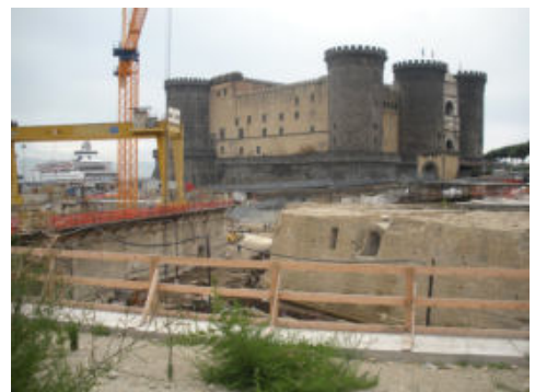
Fig. 4- Municipio square. The walls of the Renaissance citadel around Castel nuovo and the 'Incoronata' circular tower (photo by Teresa Colletta)
